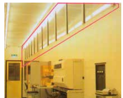
洁净室内导流垂壁 Eyelid in cleanroom
